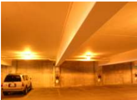
Before EverLast® retrofit, HPS Lamps stayed at full energy
