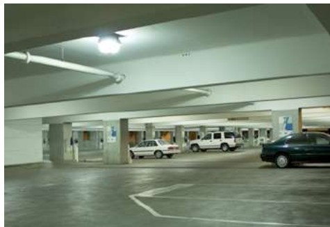
With EverLast® bi-level lighting, energy is saved when lights are dimmed and better lighting color provides for an improved visual environment
